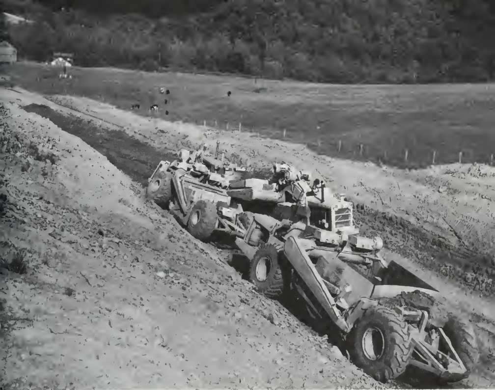
A new road is constructed in Monroe County, Ohio, as part of a rural development program.
